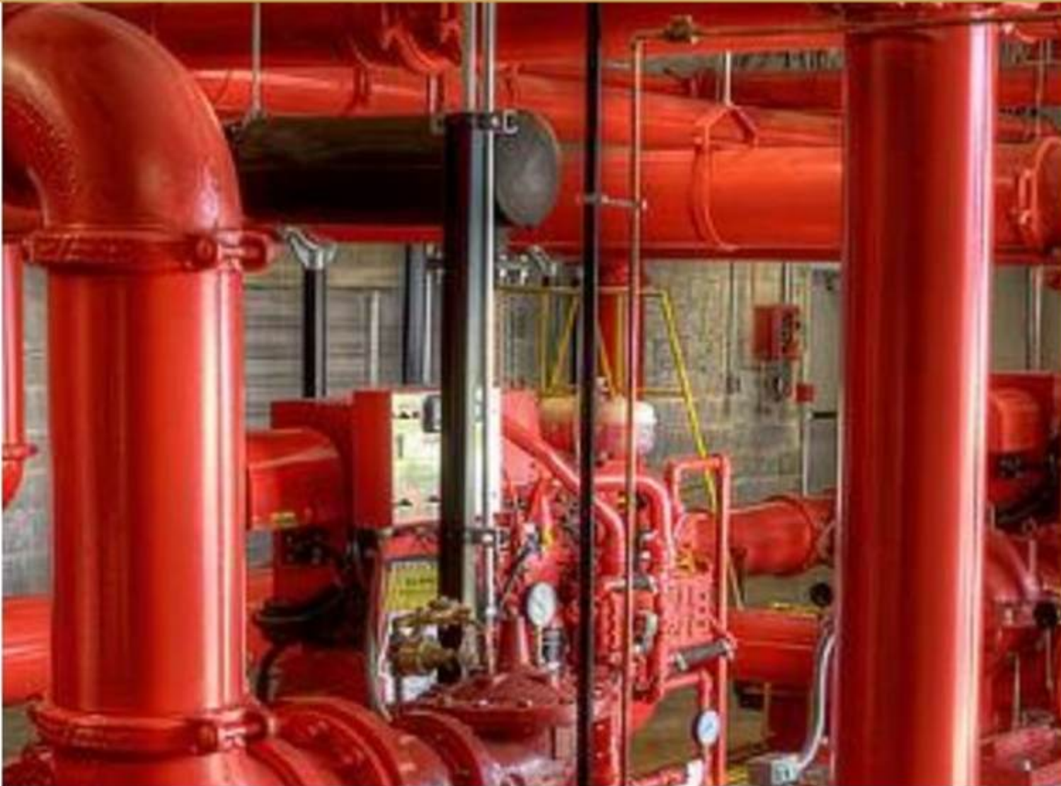
FIRE PROTECTION INSTALLATION
